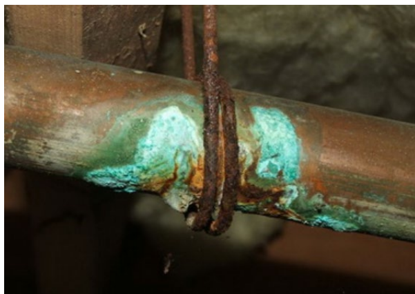
Corrosion of Copper
