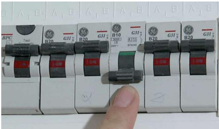
MCB (Miniature Circuit Breaker)
